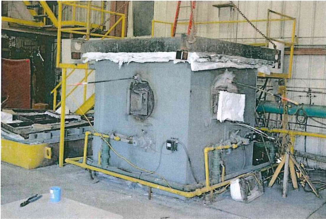
Figure B-3. Exterior View of the Furnace.
